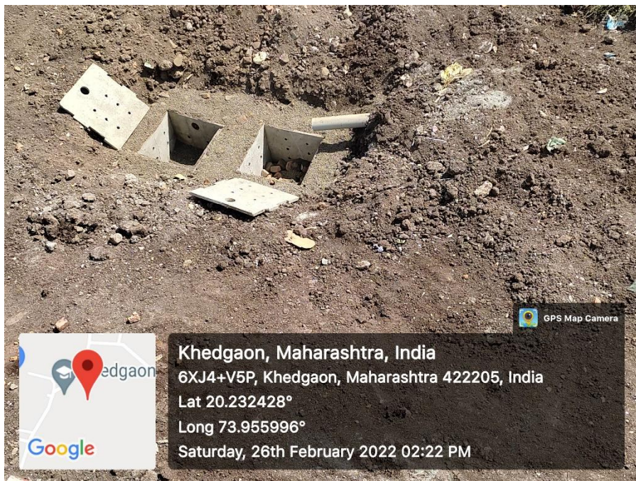
Figure 6 Picture showing rainwater harvesting pit and pipe coming through rooftop
